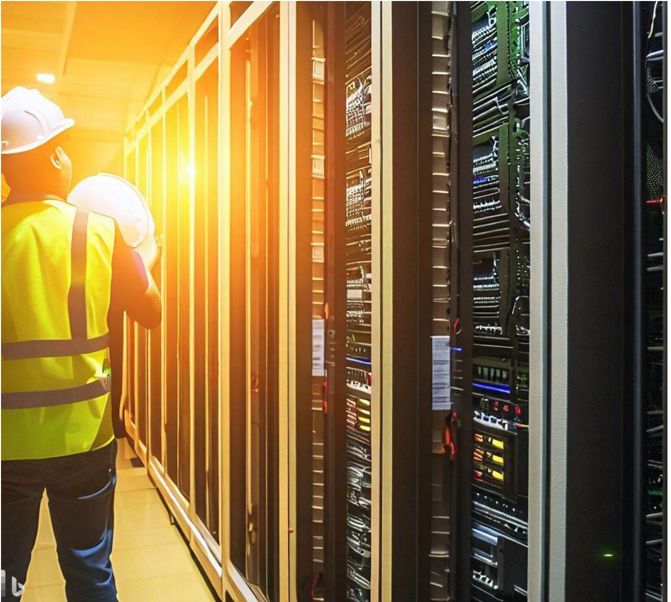
KI, Bing Image Creator: „civil engineer in server room sunset“, 17.04.23
